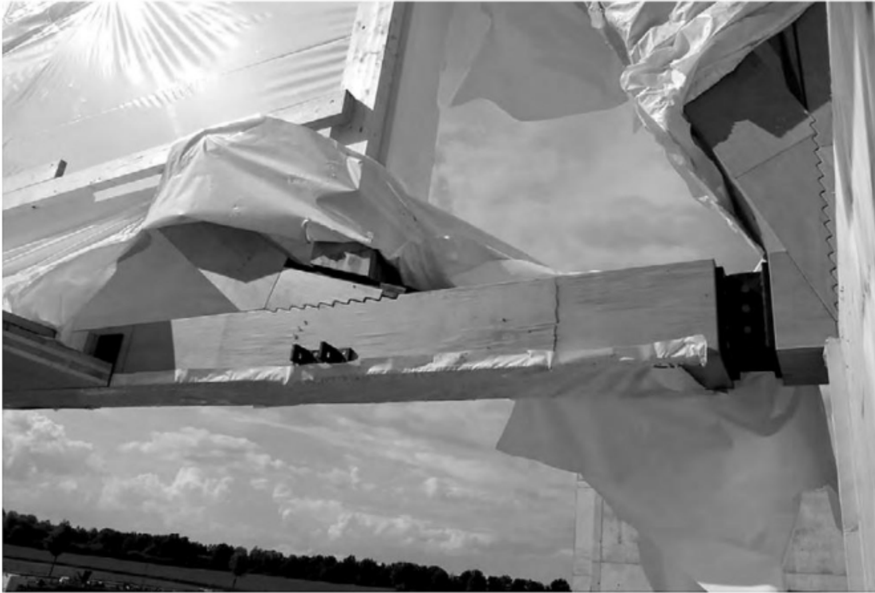
Fig. 3: Timber frame knot with 'zig-zag' joint (Hermann Kaufmann + Partner ZT GmbH n.d.).
